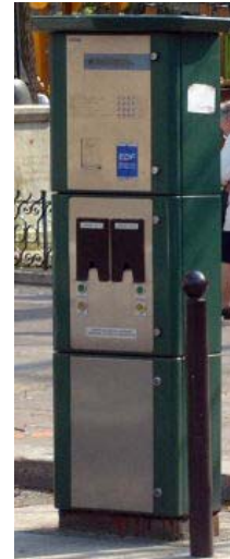
Curbside charger With payment system
