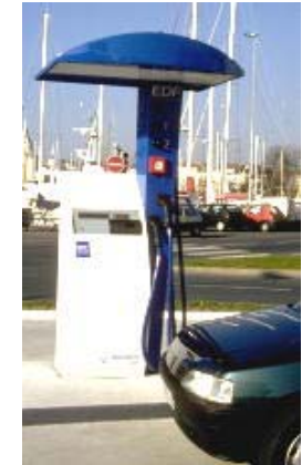
Fast charge (35 kW) (some 20 are installed)
