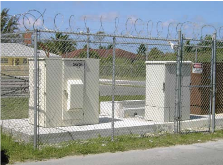
ReliOn configurable power solution - telecommunications site
