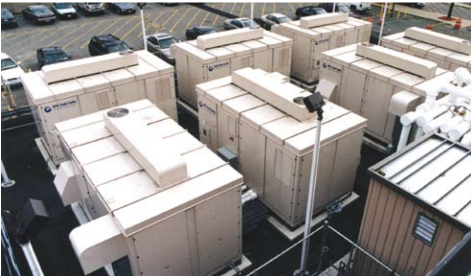
The world's largest commercial fuel cell installation – seven 200-kW UTC Power fuel cell units (1.4 MW total), installed at Verizon's calling center in Garden City, New York
