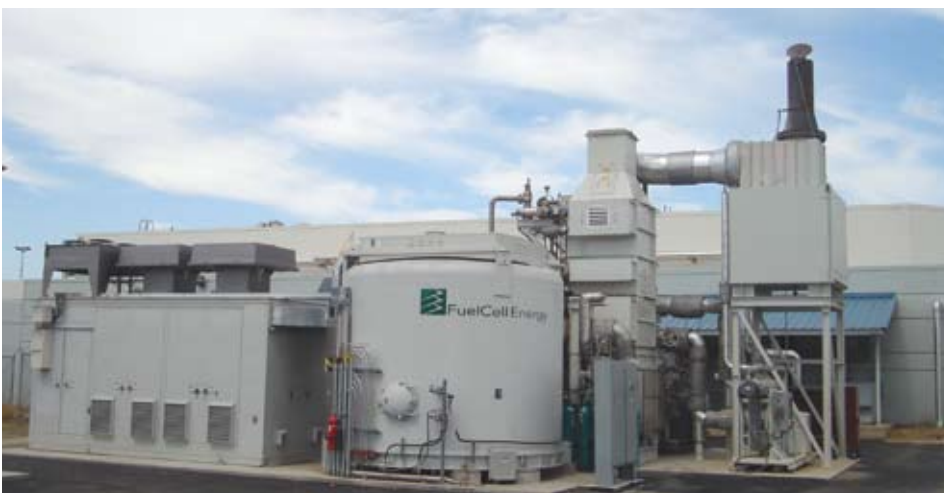
A 1 MW DFC power plant installation at Alameda County's Santa Rita Jail in Dublin, California
