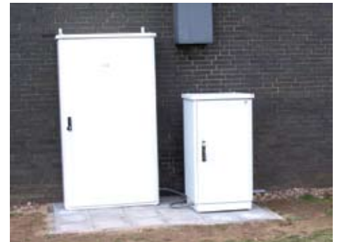
An IdaTech ElectraGen™5 installation at European telecommunications site
