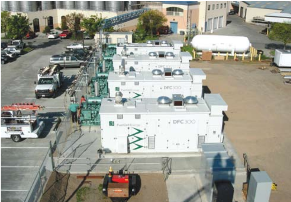
A 1 MW DFC power plant installation at Sierra Nevada Brewing Co. in Chico, California
