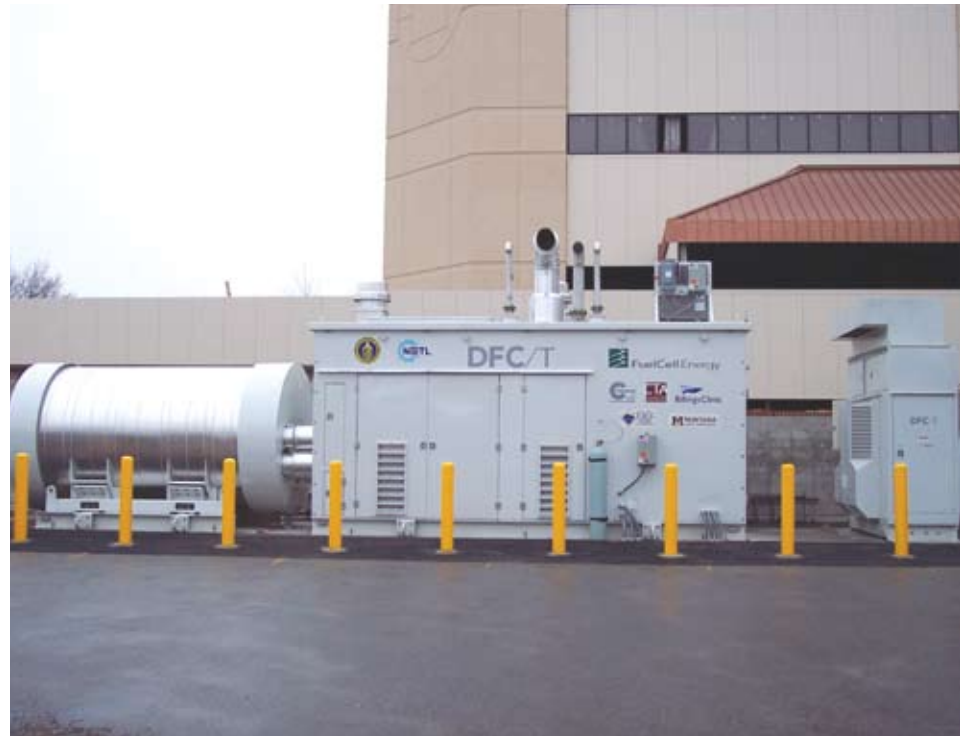
A Direct FuelCell/Turbine® installation at the Billings Clinic in Billings, Montana
