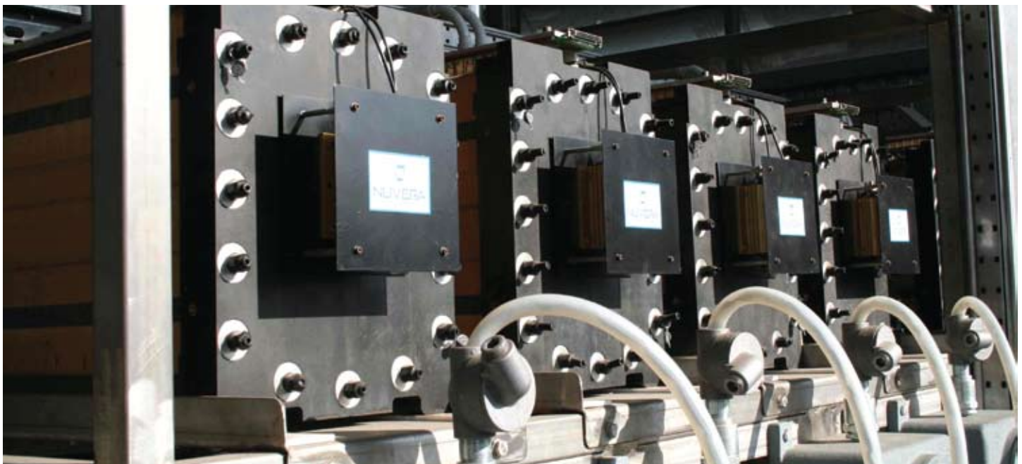
Forza modular fuel cell system installed at a customer site in Brescia, Italy
